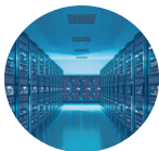
Paneles de control
